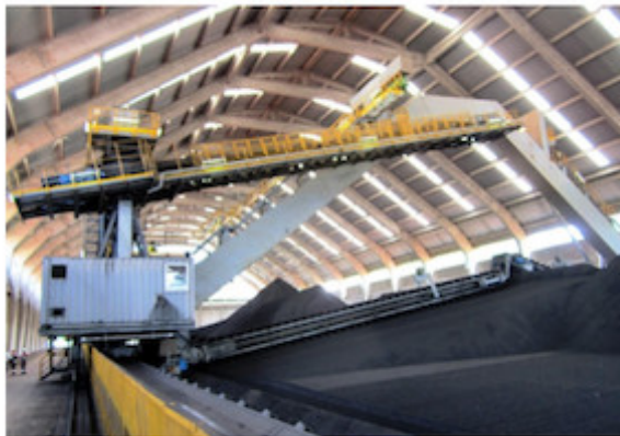
This SCHADE semi-portal reclaimer at Camp Blanco in Ecuador is typical of those installed in China (photo SCHADE)
