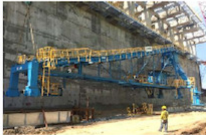
Photo 2: The Tripper Car was completely pre-assembled and lifted onto the rails with a crane. (Photo SCHADE)
